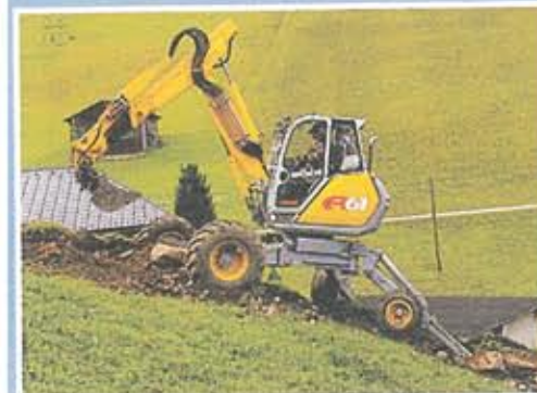
Top and Above: Good lifting characteristics, coupled with the ability to straddle the trench, make simple work of installing services in difficult terrain.
